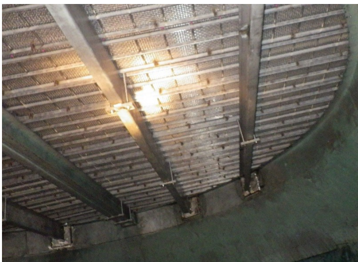
Worley Chemetics SARAMET 35 mesh pad after 4 years of operation (perfect condition)
