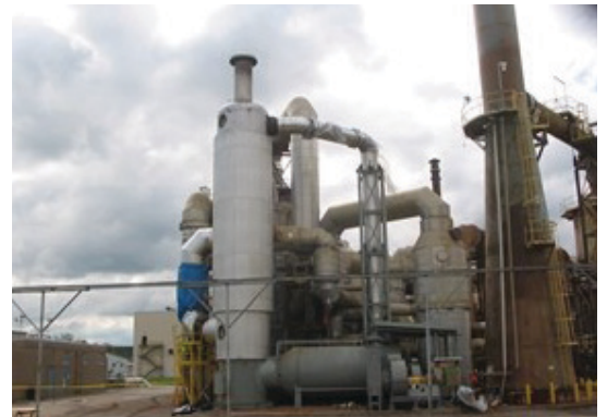
Preheat System (heat exchanger and combustion chamber) as one unit
