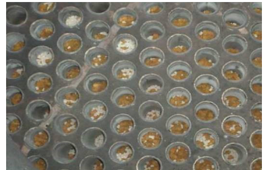
CORE™ Converter with catalyst installed (5 year inspection)
