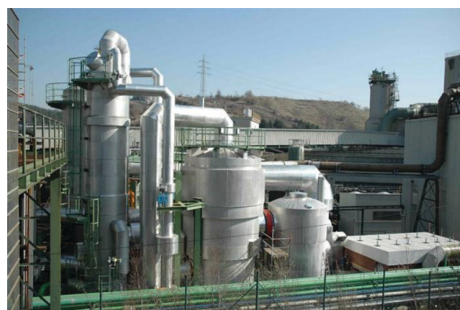
200 MTPD CORE™ Add-On System operating since 2009
